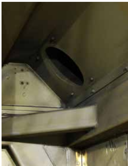
Fume extraction channels inside the cutting cell.
